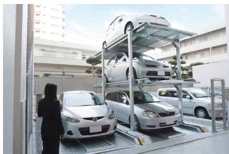
Multi-story parking equipment
