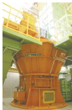
Pulverizer for non-burnable wastes
